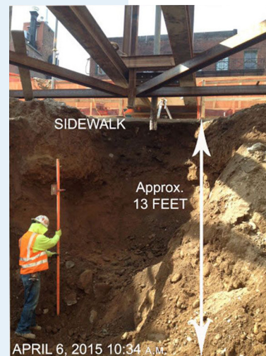
This is the trench where Carlos Moncayo was crushed to death.
